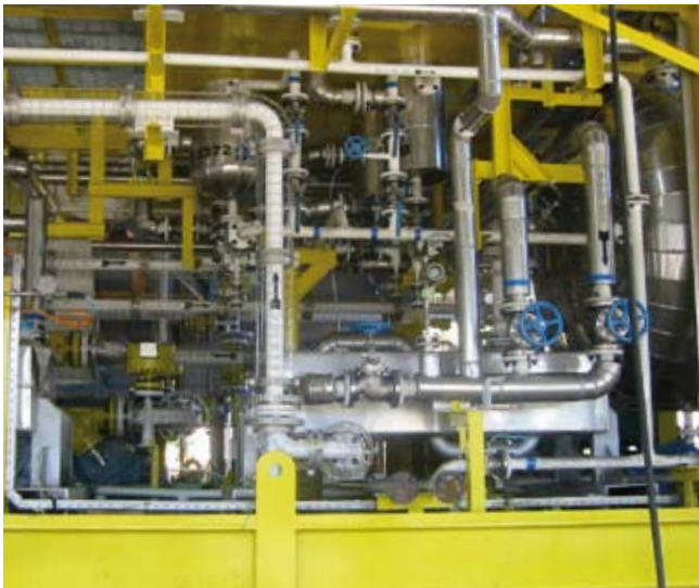
Tranter all-welded heat exchangers onboard an offshore platform.
