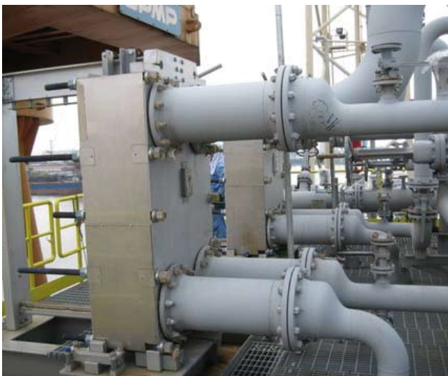
Tranter gasketed plate heat exchangers onboard an FPSO offshore Nigeria.
