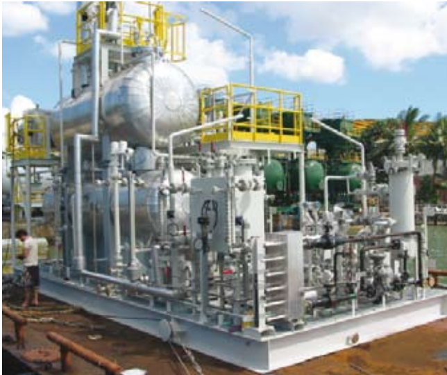
Tranter gasketed/all-welded plate heat exchangers installed on a gas dehydration skid.
