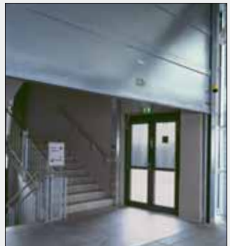
Vertical lift fire gate
