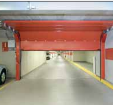
Sectional fire door
