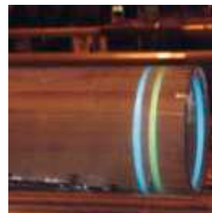
Colored ring marking on steel pipes
