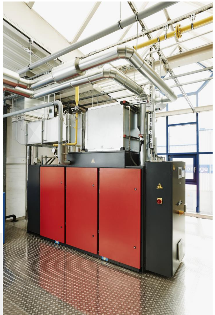
Image: Combined heat, power and compressed air system at the power station of the Bosch Thermotechnik GmbH in Lollar
